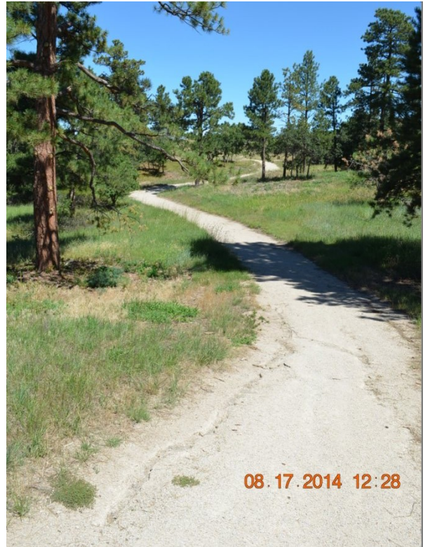
(Above): View Northward through the center of the new concrete trail project.
