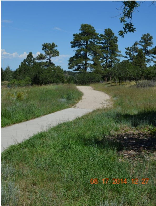
(Above): View Northward at South starting point of the new concrete trail project, at end of the existing concrete.
